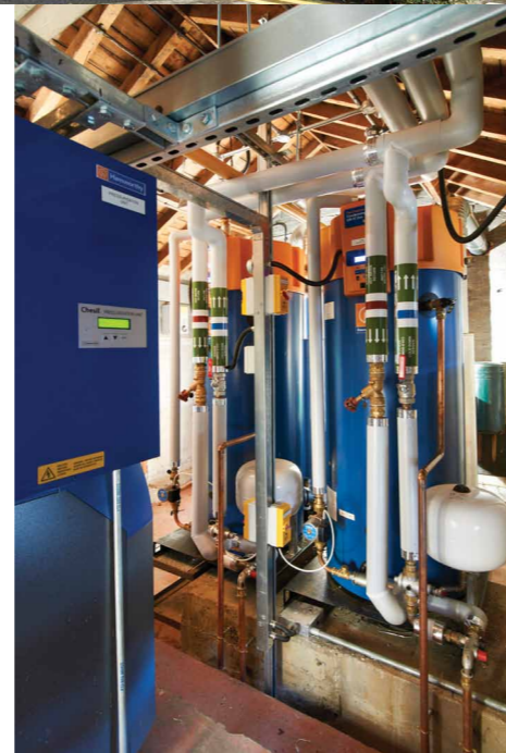
Two Dorchester DR-FC Evo condensing water heaters and Chesil pressurisation unit installed in the compact plant room at Molesey Hospital
